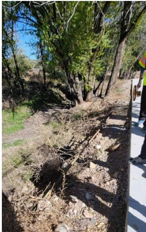
Figure 38: Sidewalk Drop-off Near Acequia Lofts
