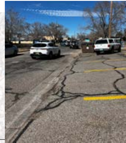
Street missing sidewalks
