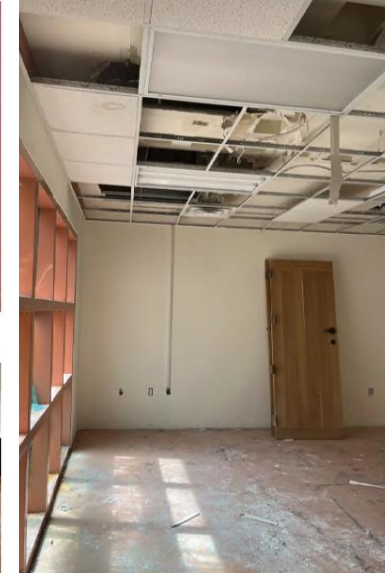
Damage to ceiling, floor, and windows, Tishman 132
