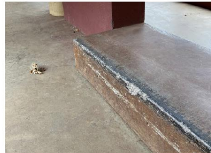
Damaged concrete bench at Marion-Tipton portal walkway.
