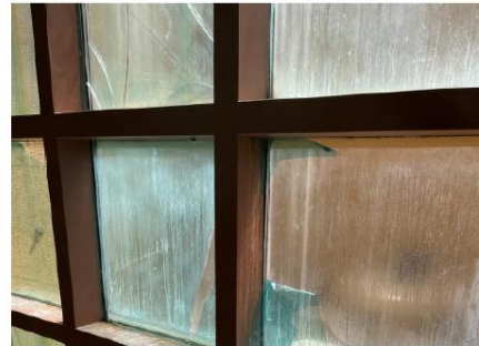
Window damage in Tishman Seminar Room 132.
