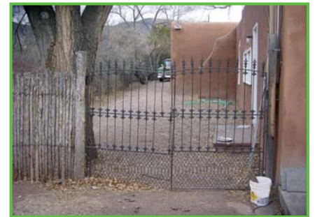
Remove sections of wood fencing that touch the house.
