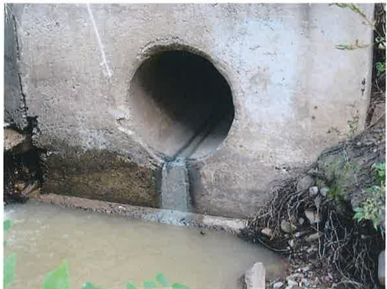
Baca Street – Illicit Discharge Connection
