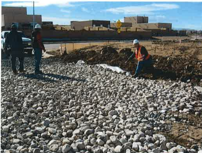
BMP Construction Entrance
