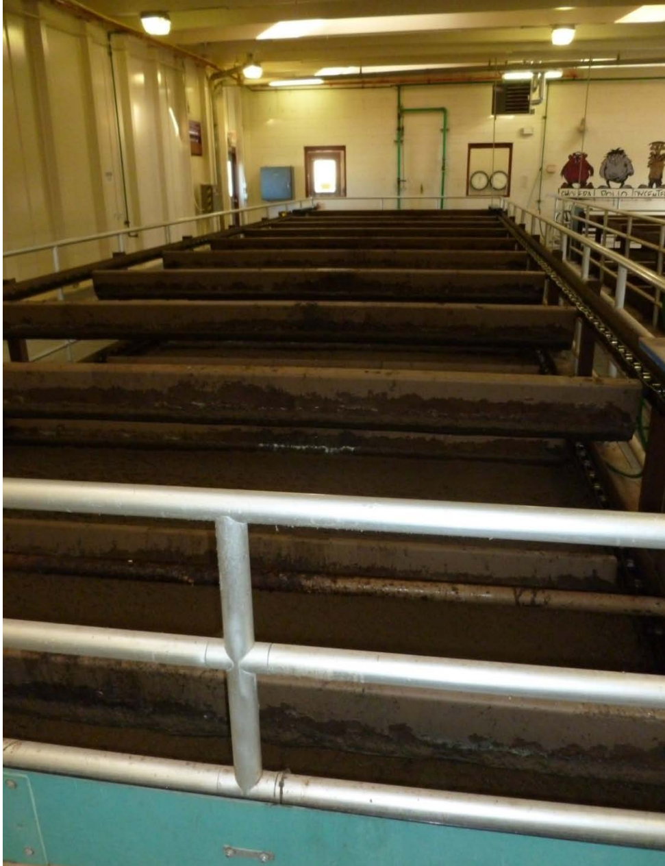
Figure 8-10. Picture of the Existing Dissolved Air Flotation Thickener
