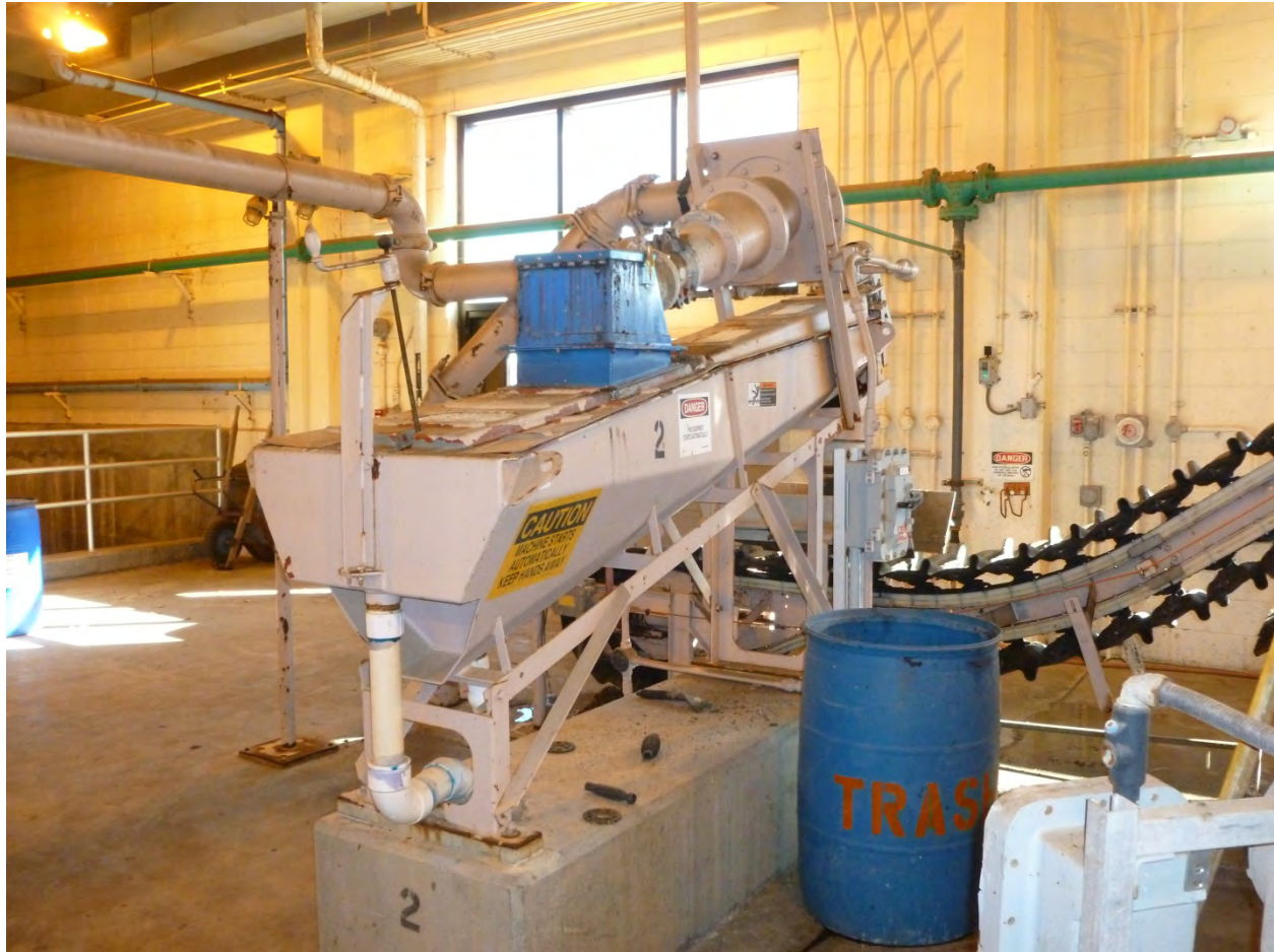
Figure 8-2. Picture of the Existing Grit Classifier Equipment
