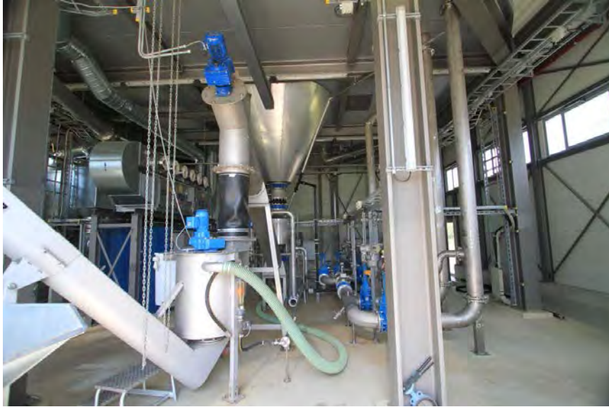
Figure 9-2: Airprex Installation in Berlin, Germany
