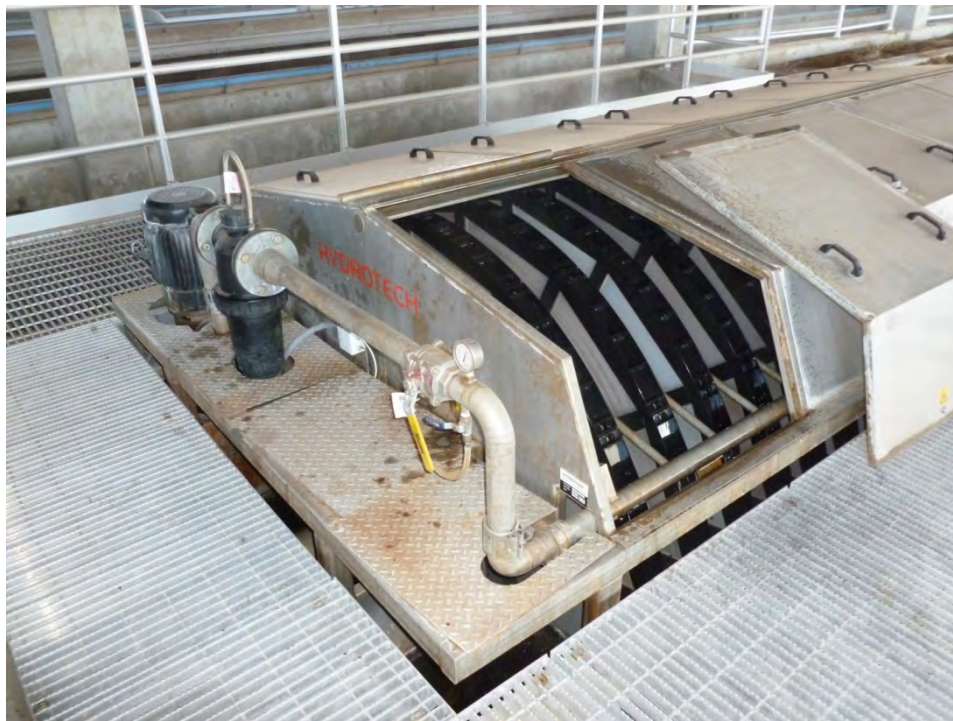
Figure 8-6. Picture of the Existing Disk Filtration Equipment
