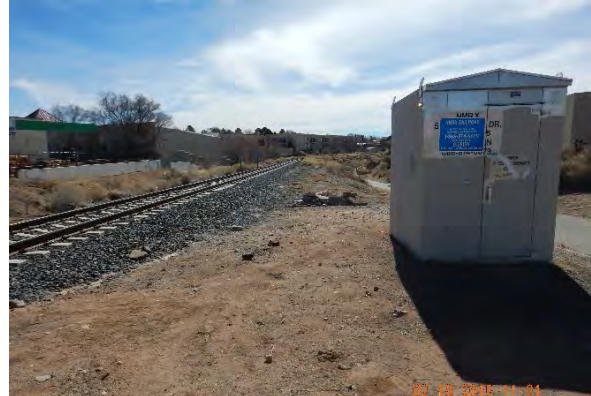
Figure 6. Railroad Controller Bungalow
