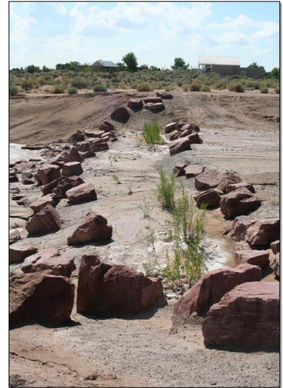
Photograph: Grade control structure in the Lower Montoyas arroyo incorporating planting strip. (Source: SSCAFCA)
