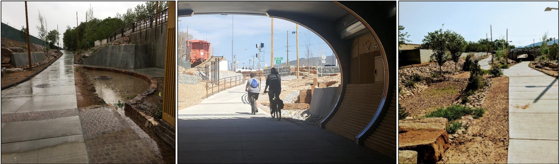
Photographs: The completed Acequia Trail Underpass project (Source: City of Santa Fe).
