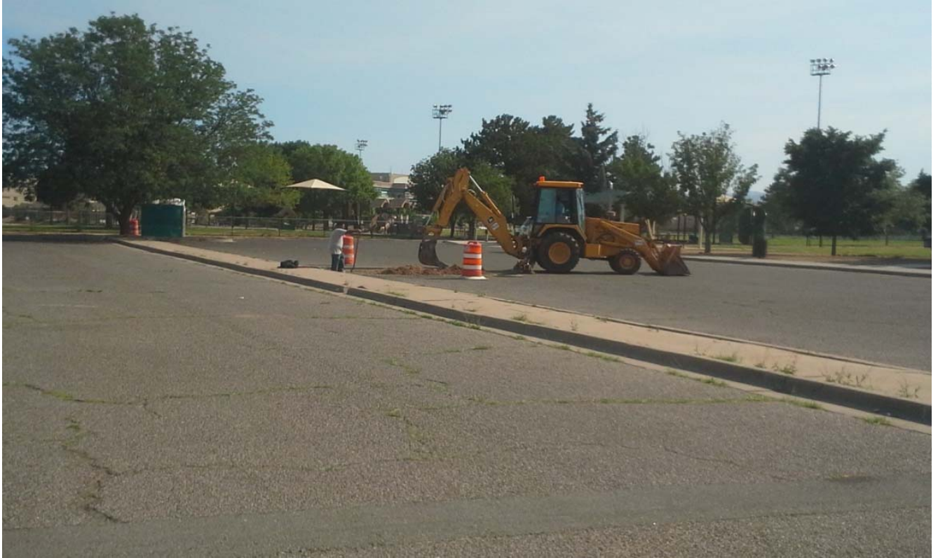
Pavement from underutilized parking spaces being removed in General Miles Park and replaced with rain gardens to promote infiltration. (Photo credit: Santa Fe Watershed Association)
