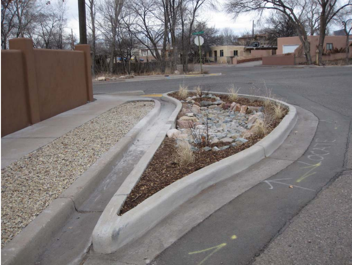
A small bioretention system was constructed in 2016 by retrofitting an existing vacant curb median at the intersection of Espinacitas and Hopewell streets in Santa Fe. (Photo credit: Santa Fe Watershed Association).
