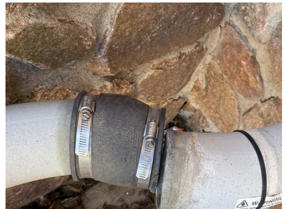
Fire water line is detached | A25
