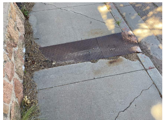
Plate over drainage | A7
