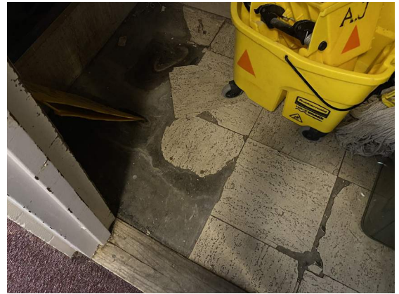
Poor condition VCT in janitor closet | A9
