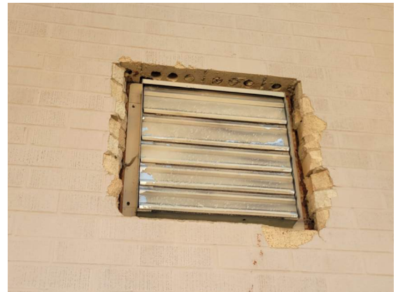
Damage at exterior louvre | A5
