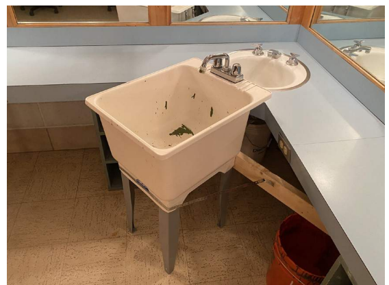
Dressing room retro-fitted sink | A23
