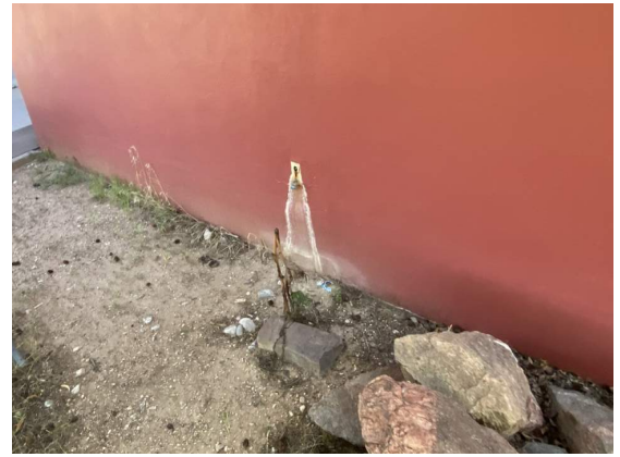
Water connection on exterior | A24
