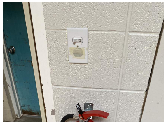
Older light switch with taped outlet | A26
