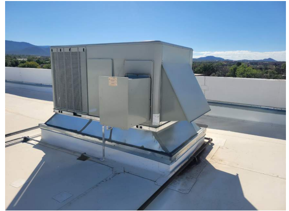
Roof-top package units | A20
